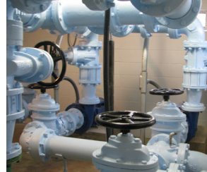
Water Pump Stations
