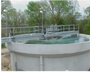
Water Treatment Plants
