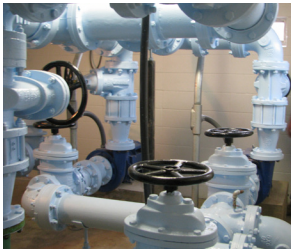
Water Pump Stations
