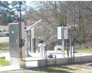
Wastewater Lift Stations
