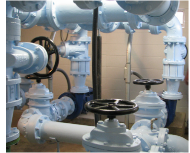
Water Pump Stations
