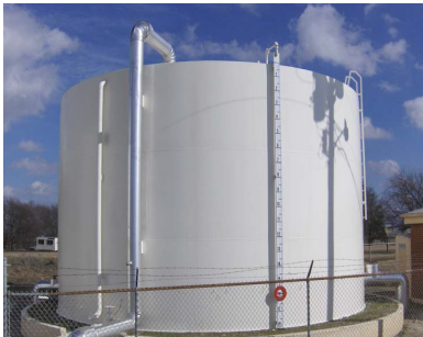
Water Storage Facilities
